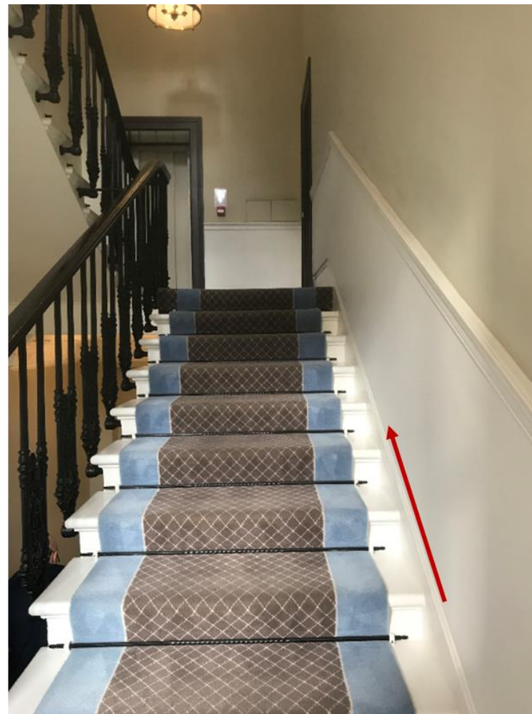
InvisiLight 12f in corridor along stairwells
